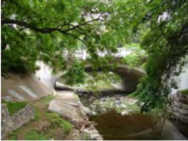
Paths along the creek are discontinuous and in poor condition.
